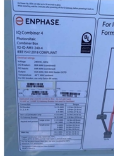
The entire inverter label is visible and legible in the photo.
