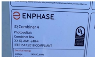
Only a portion of the inverter label is visible.
